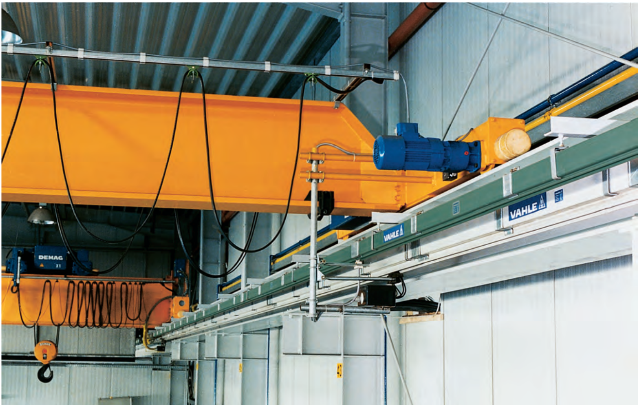
Powerail for the current supply of a hangar crane.
